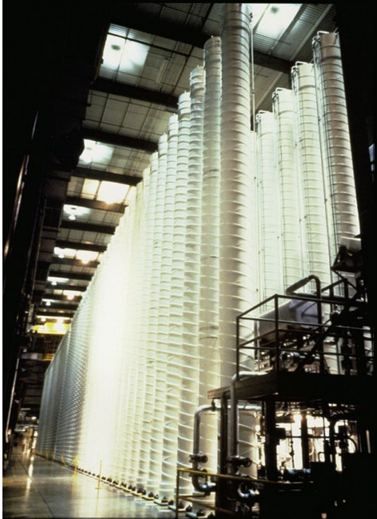
Figure 71. Gas Centrifuge Cascade at K-25
